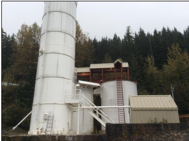
Water Treatment Plant
