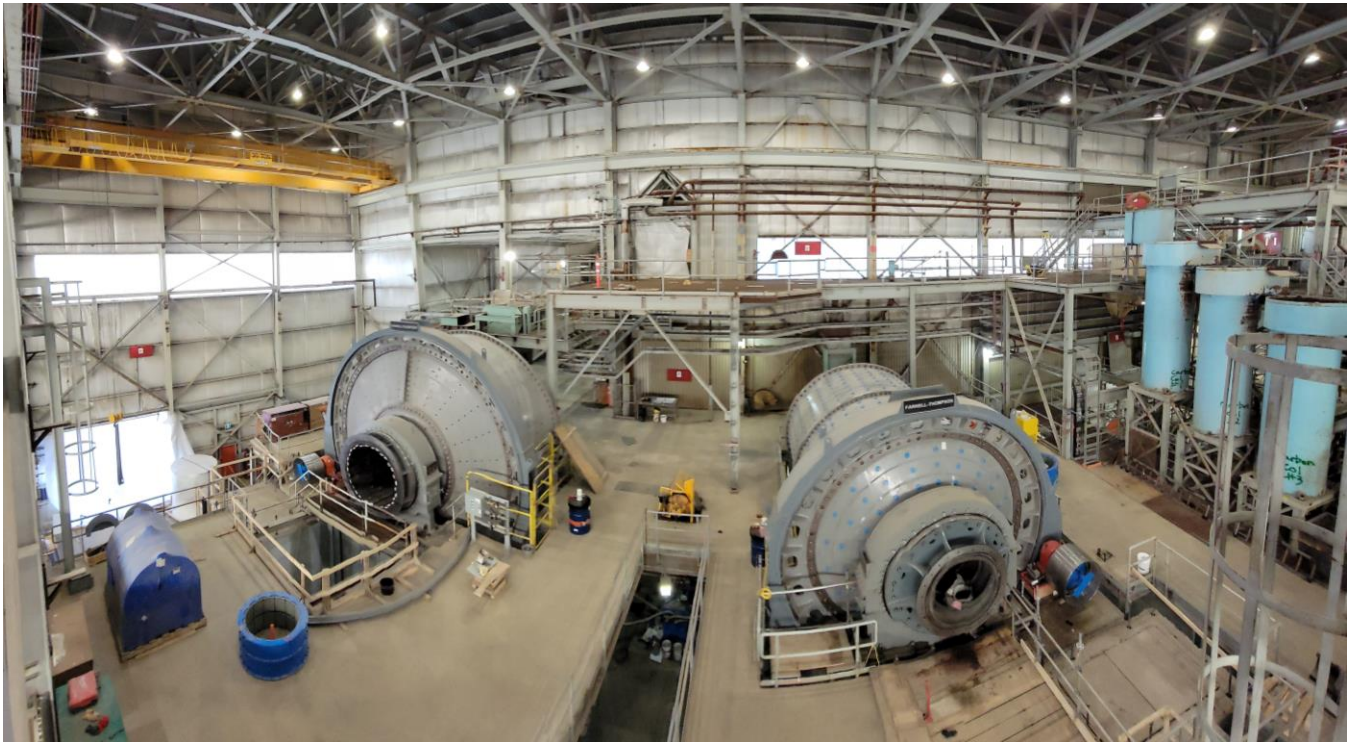
Figure 1 – Interior of mill building showing SAG (left) and Ball (right) mills installed
