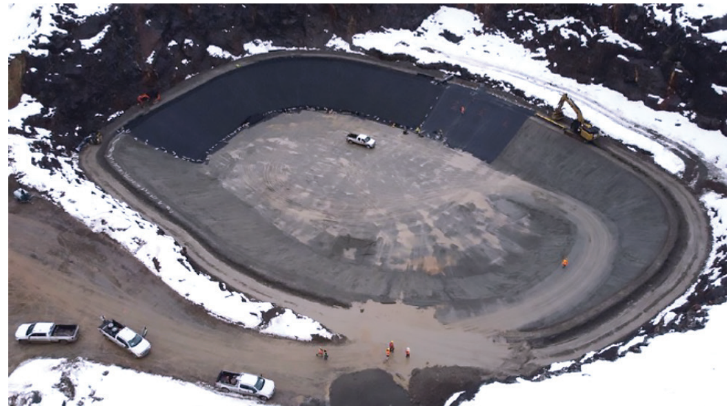
Construction of the water retention pond for waste water from underground mining to be treated by the water treatment plant
