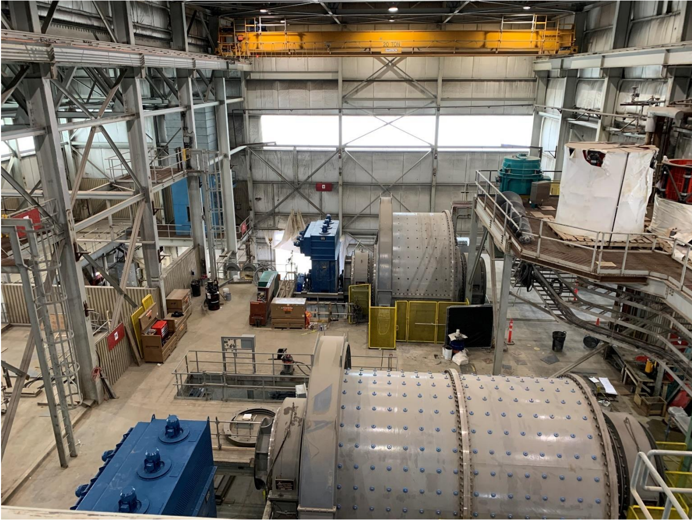
Figure 5 – Mill building interior showing Ball and SAG mills with motors installed
