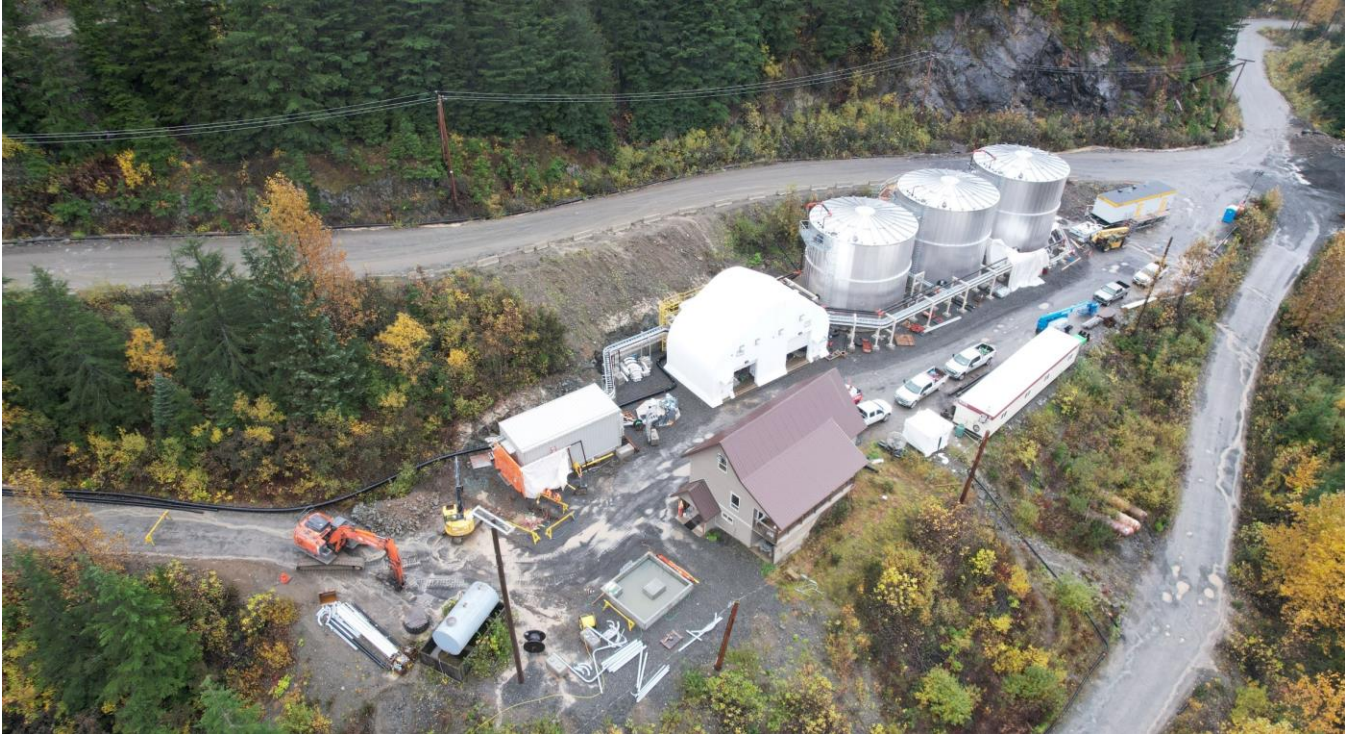
Figure 4 – New WTP MBBR tanks and electrical building
