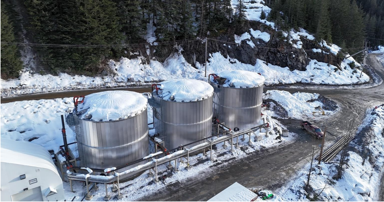
Figure 5 – WTP MBBR system
